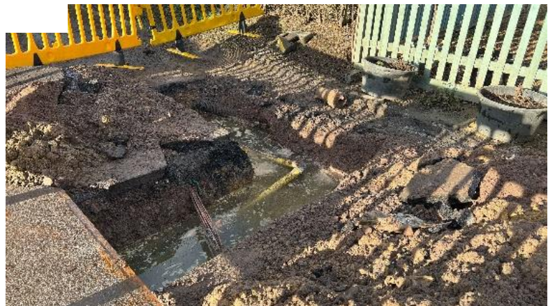
Figure 10 Infiltration affects all underground pipework. Here the gas main contains water.
