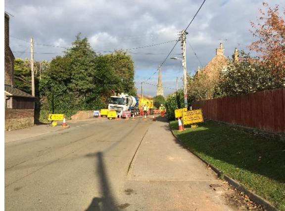
Figure 11 Severn Trent works to grout sewer pipes in St John's Road and Churchend
