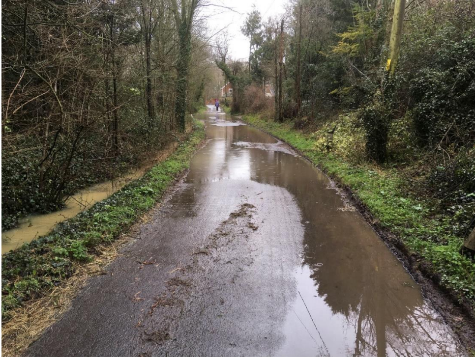
Figure 5 Flooding in Ryalls Lane February 2020. The ditch is full and cannot drain the road.
